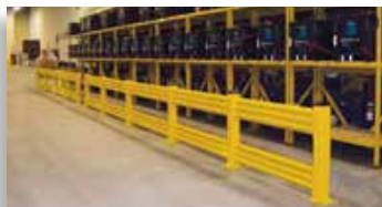
Guarding battery racks
