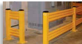
Guarding electrical panels
