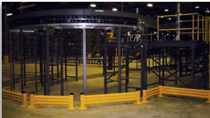
Guarding overhead conveyor
